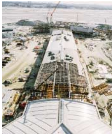
Once complete, Pier F will accommodate international operations offering passengers retail and concessions that reflect the international travel experience.
