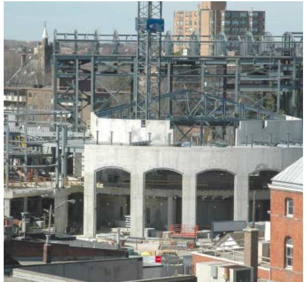
Construction is progressing rapidly on the new Performing Arts Centre in downtown Brampton.
